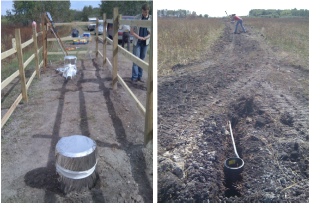
Figure 2. Backbone MT Array field equipment installed in NW Minnesota, USA. Magnetometer and data acquisition systems are buried in 2-m deep underground vaults; electric dipoles are typically 500 m long, terminated in electrodes buried 1 m deep in large volume of double-saturated NaCl/kaolinite paste. Systems are solar powered and telemetry is being implemented. The backbone installations are planned for 5-year deployments or longer, yielding a period range of 10 s - 100,000 s.
